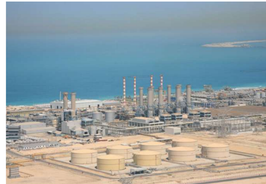
Fig. 26. A desalination plant in Shaiba, Saudi Arabia (Aramco)
