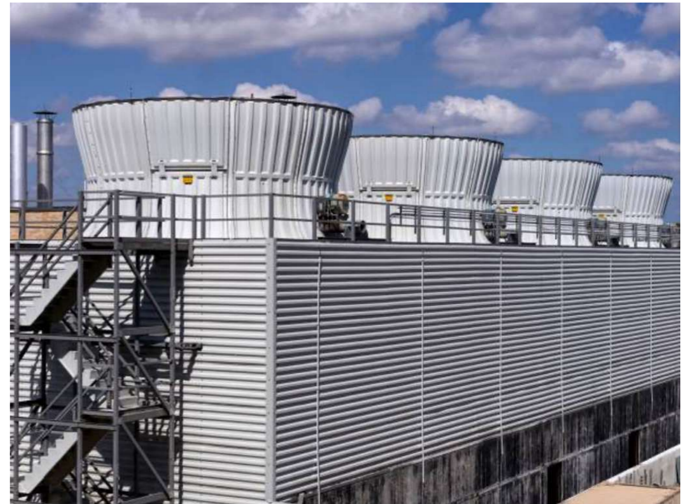
Credit: Sustainable District Cooling Systems: Status, Challenges, and Future Opportunities, with Emphasis on Cooling-Dominated Regions
